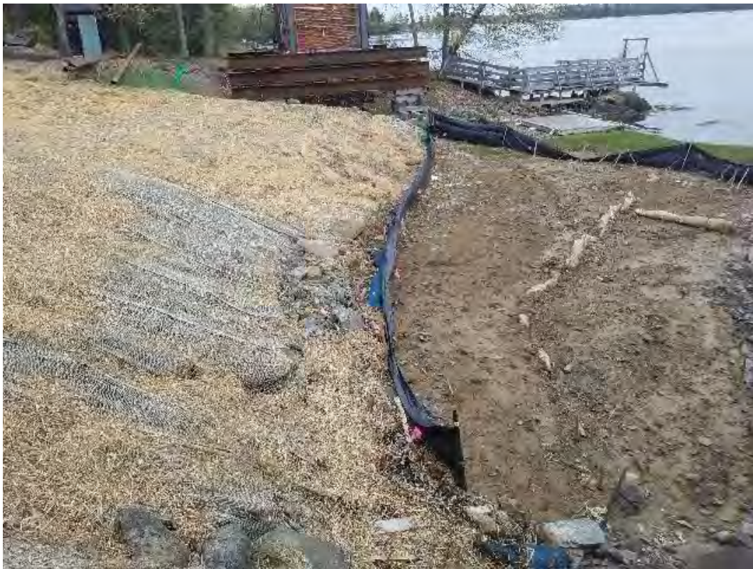
Fig 10: Settling of material for salt marsh restoration at Getchell property/west side of the Bay. Viewing north. (05-18-20).
