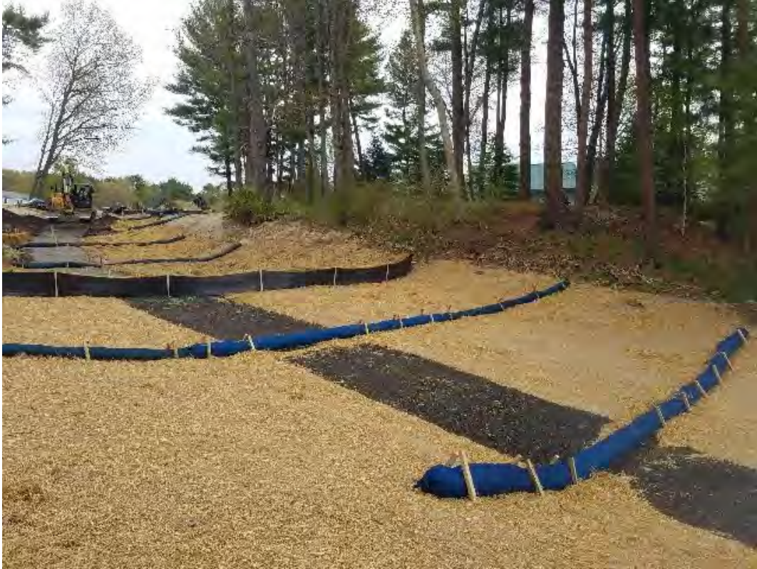
Fig 5: Restoration of slope at Gundalow landing/east side of the Bay. Viewing east. (05-15-20).
