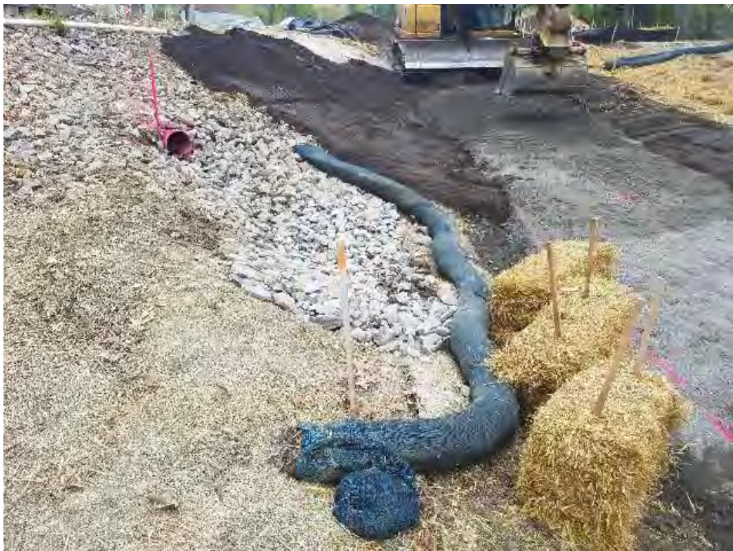
Fig 4: Repaired existing drainage culvert and rip rap swale along slope at Gundalow landing/east side of the Bay. Viewing east. (05-15-20).
