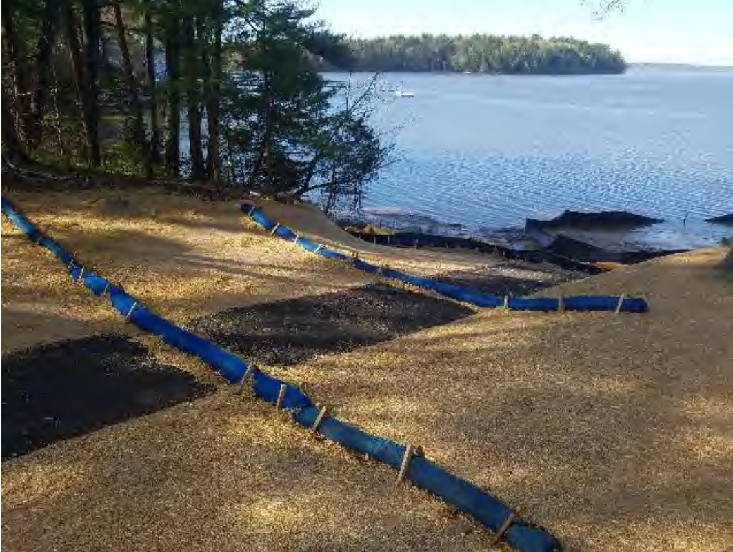
Fig 3: BMPs on slope below manhole at Gundalow landing/east side of the Bay. Viewing southwest. (05-14-20).
